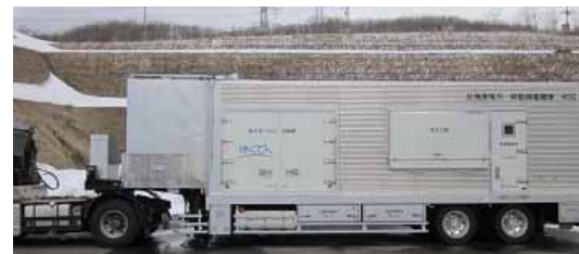
Power generation vehicle (deployed since March 2011)
