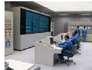
Thermal power plant operation simulator
